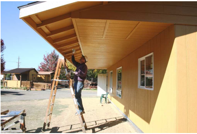
(LEFT) Although most of the Mack Walch library building was painted by the Walch family and friends in September, there remained a few small areas left to do. Here Rick Aubin is applying paint to underneath the roof overhang. — Tony Johnson photo
