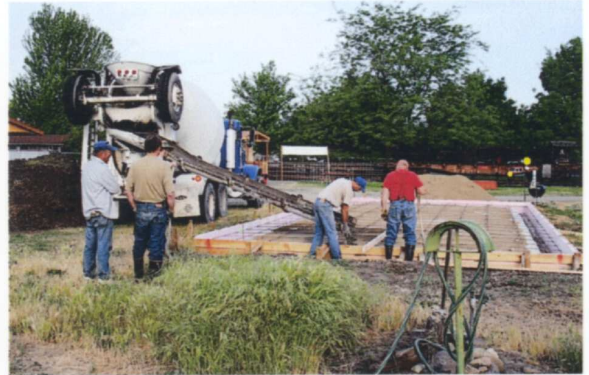
The first truck arrives five minutes early. The first pour is where the back wall will sit; then we followed along the forms, filling in the north side of the building first. — Tony Johnson photo
