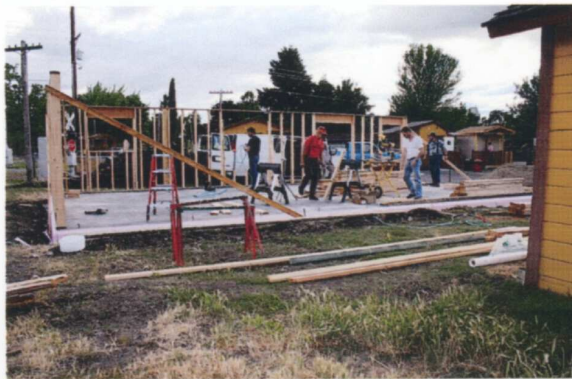
It's getting near the end of the day, the boys have secured the walls for the night, and it's time to secure the tools. — Tony Johnson photo
