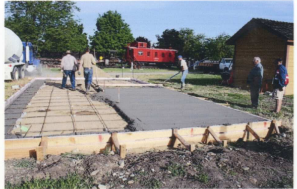
It's a little after 8:00 am and nearly half the foundation is poured and leveled. We didn't run into any unforeseen problems that day. — Tony Johnson photo
