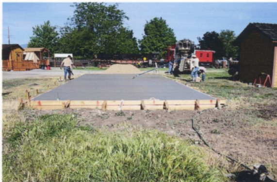
At 9:40 am we finished pouring the foundation. Next will come the scraping and smoothing of the slab. — Tony Johnson photo
