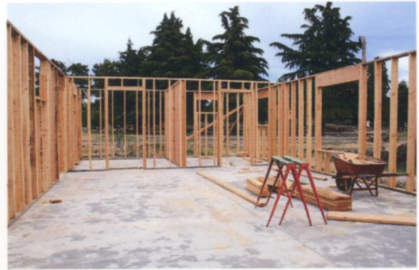
This is how far along the building looked by June 1. The four exterior walls, plus the walls for the two offices, are in place. Currently we are checking the price on trusses. — Tony Johnson photo
