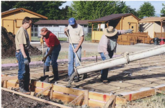
Larry Tuttle (far left) carefully watches the concrete mix as it pours into the forms. John Powell (far right) motions to the driver to move ahead slowly. — Tony Johnson photo
