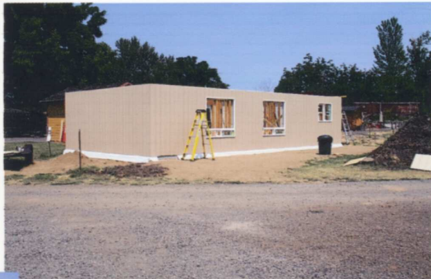
(RIGHT) All done! To save time we didn't fully nail the siding in place; instead choosing to do it after all the siding was properly in position. Jerry finished nailing the siding a few days later. — Tony Johnson photo
