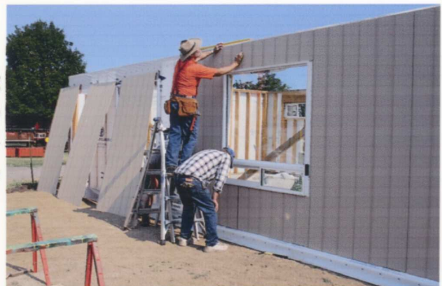
(RIGHT) Ric and Steve hold the siding in position as Jerry uses a level to guide the panel so it will both fit perfectly with the adjacent panel and be absolutely level. — Tony Johnson photo
