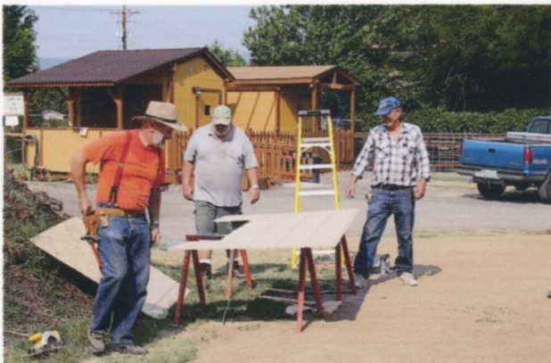
(LEFT) With Jerry Hellinga in charge this day, Ric Walch and Steve Bruff are ready to lift an already cut panel of siding into position. Also helping this day were Tom Baldwin, Rick Aubin and Tony Johnson. — Tony Johnson photo
