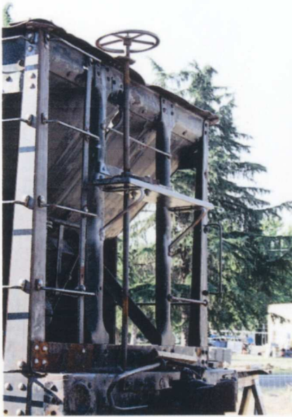
(LEFT) Not to be overlooked with all that goes on at the Railroad Park, is all the restoration work Steve Bruff is doing to our Pacific & Eastern Railroad hopper car. In this photo the repaired brake wheel and stand is back in position, plus a new brakeman platform has been installed; replacing the old wooden platform that rotted away decades ago. — Tony Johnson photo
