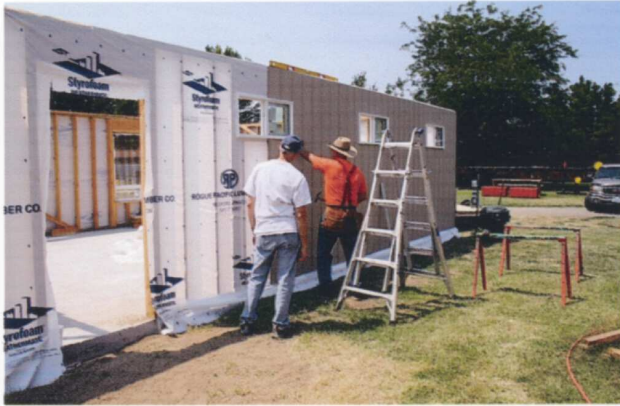
(LEFT) With the South and West sides of the building done, Tom Baldwin and Jerry work on the North side. I would estimate it took us about four hours to hang and nail all the siding in place. — Tony Johnson photo
