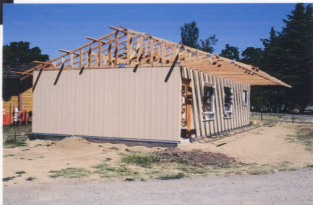
(RIGHT) This is how the building looked as of press time. Out of sight in this photo is our chapter truck with a load of roofing and tarpaper. In a few weeks it'll be installed and then we'll turn our attention to the interior. — Tony Johnson photo
