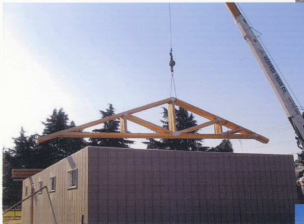
(LEFT) The big day came on July 26 when the roof trusses were delivered. In this shot a batch of trusses is lifted on top the building. Work on erecting the trusses in place began as soon as they all were unloaded. — Rick Aubin photo
