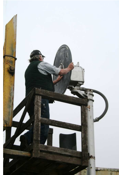
(ABOVE) Randy uses our chapter's special forklift platform so he can easily remove signal parts and install the new lens.
