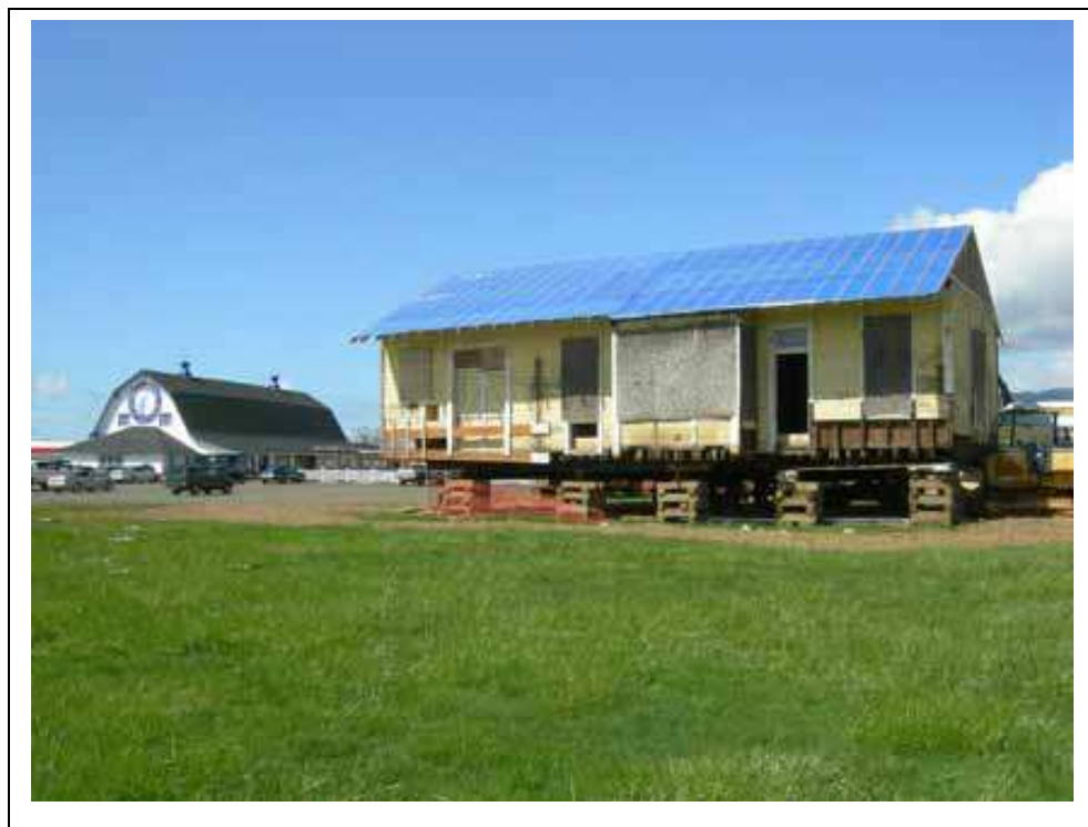
At its new, permanent location at the Blue Heron French Cheese Company facility, the depot still needs a new foundation and replacement roofing.
