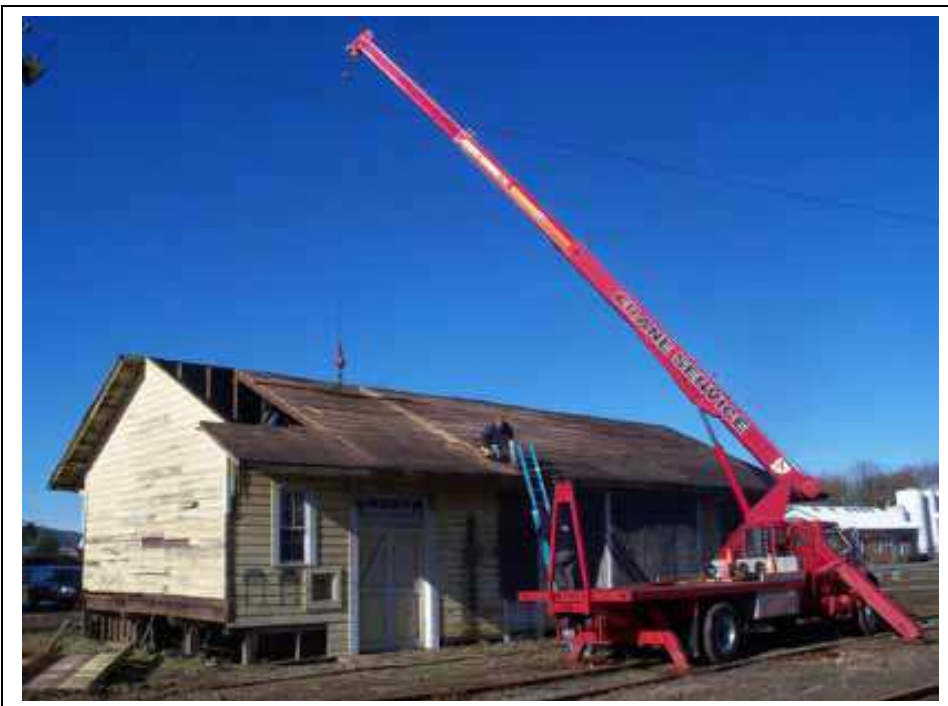
In preparation for the move, the roof of the depot had to be removed. A crane allowed the clean removal of all of the roof joists and covering.
