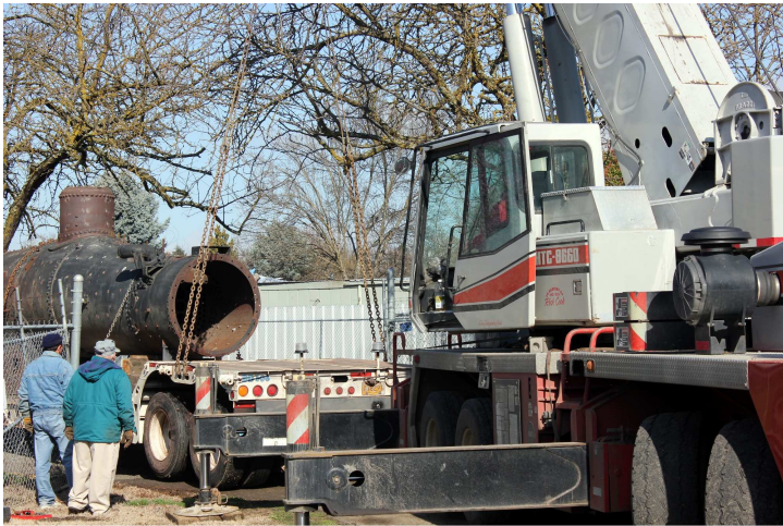
The crane had to be used to “slide” the back of the trailer Sideways to clear the gate.
