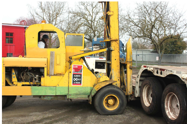
Above: Jerry is lifting and sliding the trailer so the trailer can be backed under the boiler. Check out that front tire.
