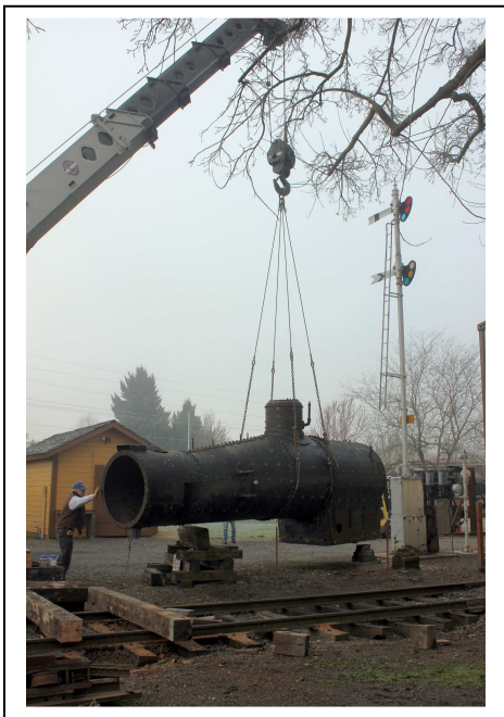
Left: Jerry is assisting the crane operator to keep the boiler from spinning while it is being lifted.
