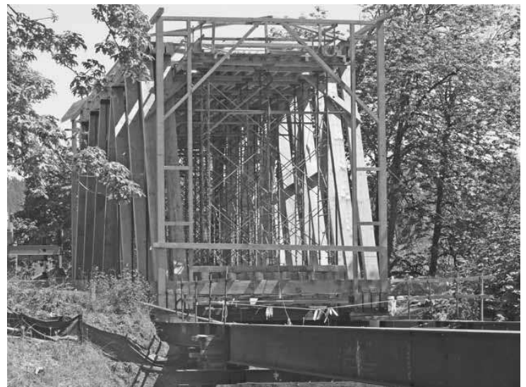
Above right: By August 2011, the framing for the bridge ends had been constructed and the roof rafters were being installed. The beams in the foreground are launching rails to permit the bridge to be pulled across the river and seated on its foundations. All photos, Kent Hutchens
